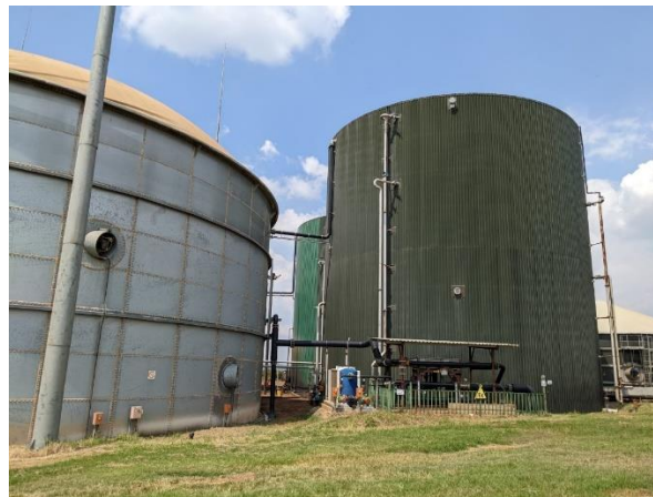
Figure 26: Bronkhorstspruit Biogas Project
