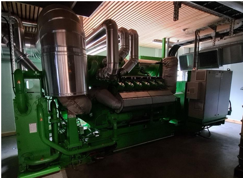
Picture 25: CHP unit to produce combined heat and power from wood gas
