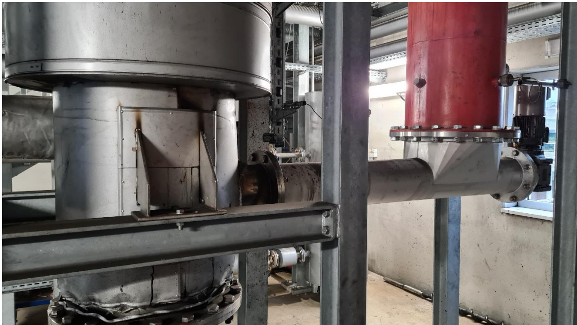
Picture 9: Intake auger screw into an upstream gasifier
