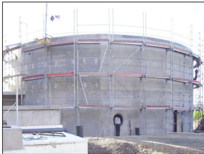
Picture 22: Concrete digester.
