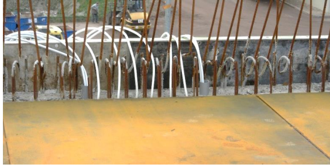
Picture 29: Heating system with floor heating pipes directly integrated into the concrete wall.
