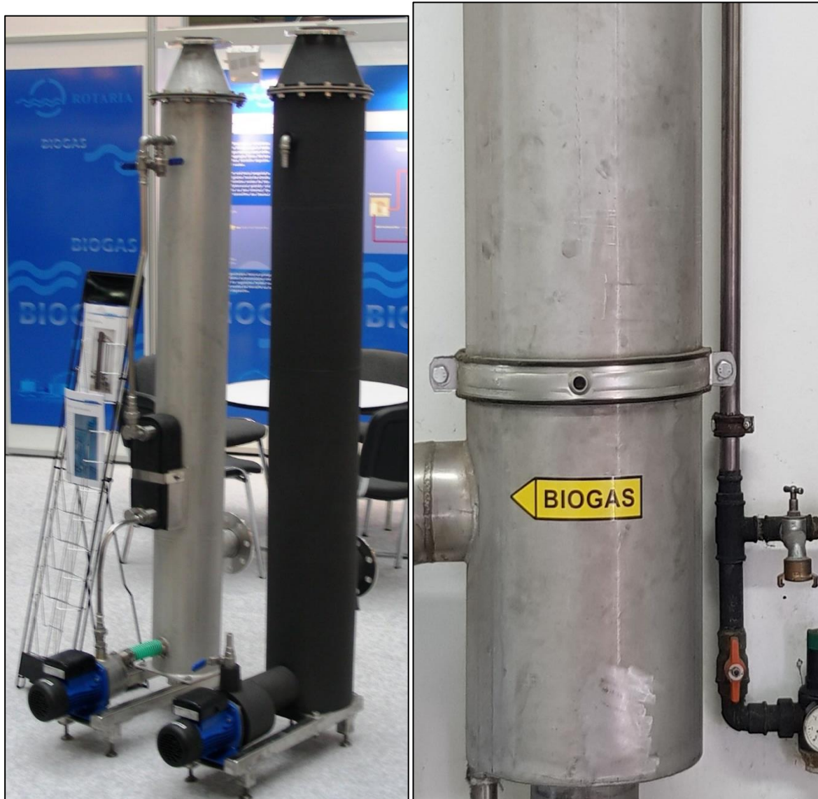
Picture 67: External biogas coolers with integrated particle separator.
