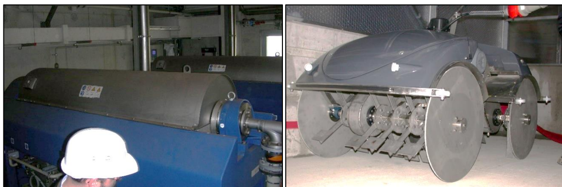
Picture 52: Left: decanter, right: automatically driven digestate turner.
