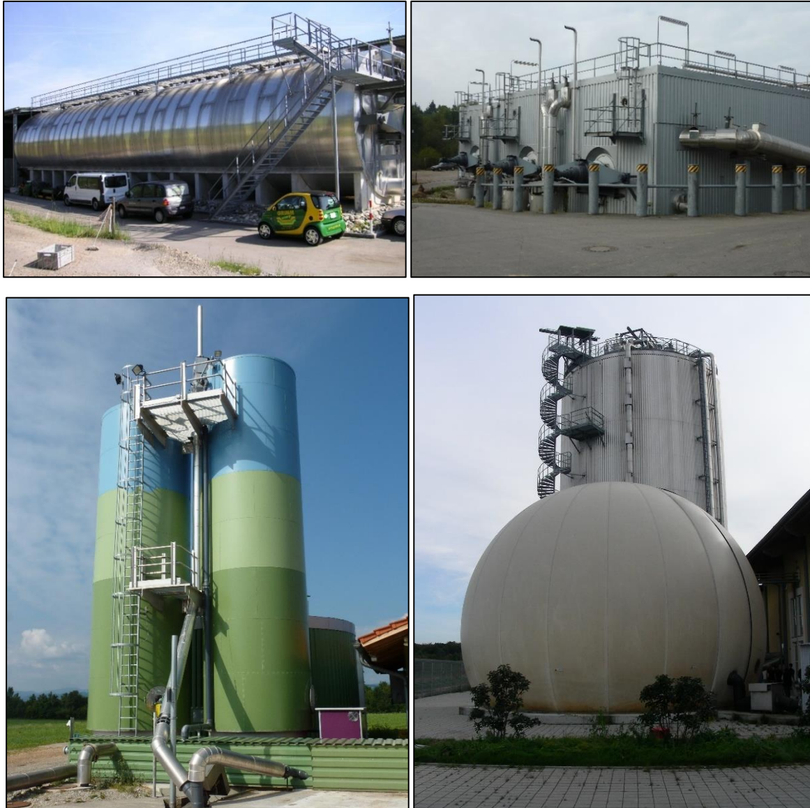
Picture 17: Top: Horizontal dry digester with horizontal stirring (left round and of steel, right: square and of in situ concrete - digesters in parallel), bottom left: upstream plug flow digester without stirring, bottom right: downstream plug flow digester without stirring (in the background).
