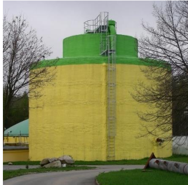
Picture 16: Hydraulic digester with the higher inner tank and the lower outer tank.
