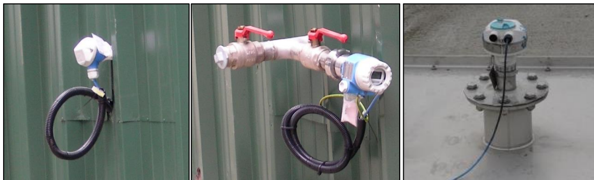
Picture 46: Measurement devices for temperature and level sensors (right: ultrasonic measures from top).
