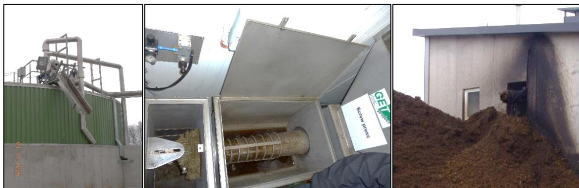
Picture 51: Screw press to dewater digestate.
