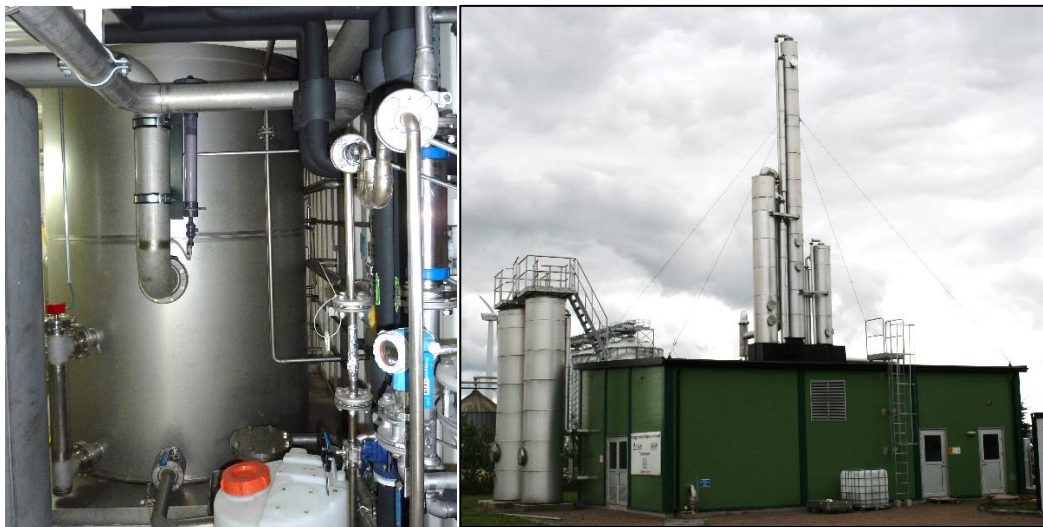
Picture 71: CO 2 separation through physical scrubber, left: scrubber column, right: physical scrubber installed in a container.
