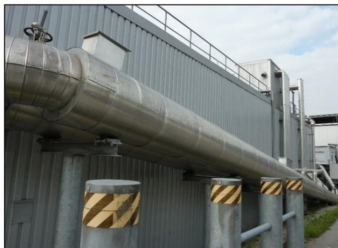
Picture 31: External heat exchanger where the substrate that will be fed gets heated and pressed into the digester.
