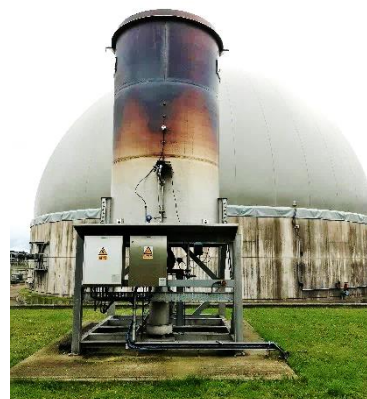
Picture 43: Enclosed flare in biogas plant.
