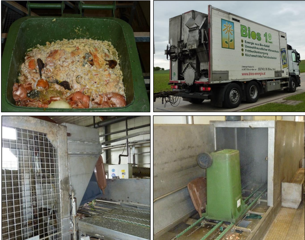
Picture 5: Top left: organic waste bin from catering and households, right: collecting lorry for catering and household waste with integrated emptying and cleaning device, bottom: organic waste bin emptying facility at the biogas plant with a subsequent washing-bay.
