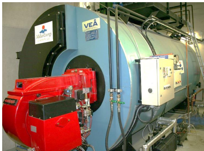
Picture 69: Typical peak load boiler for biogas with a capacity of 7.2 MW th .
