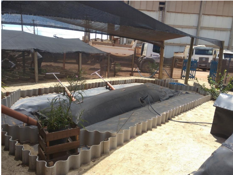
Picture 74: Plastic bag digester, Source: Ökobit
