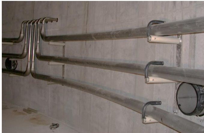
Picture 30: Stainless steel heat pipes directly attached to the digester wall. To avoid corrosion stainless steel pipes need to be installed galvanically isolated.
