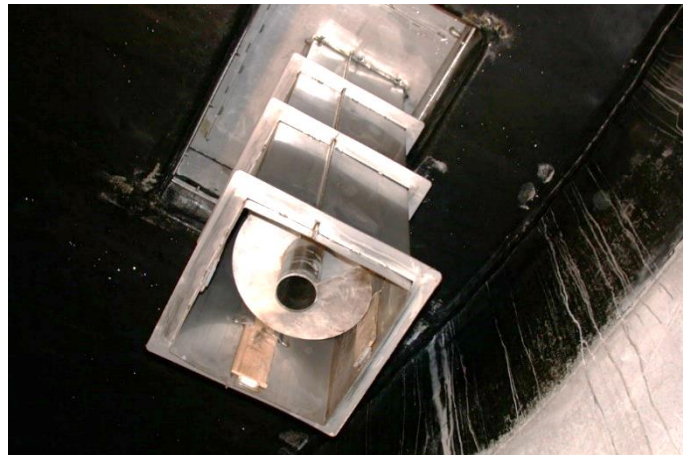
Picture 11: The feeding screw must always end below the liquid surface so that no biogas can escape.
