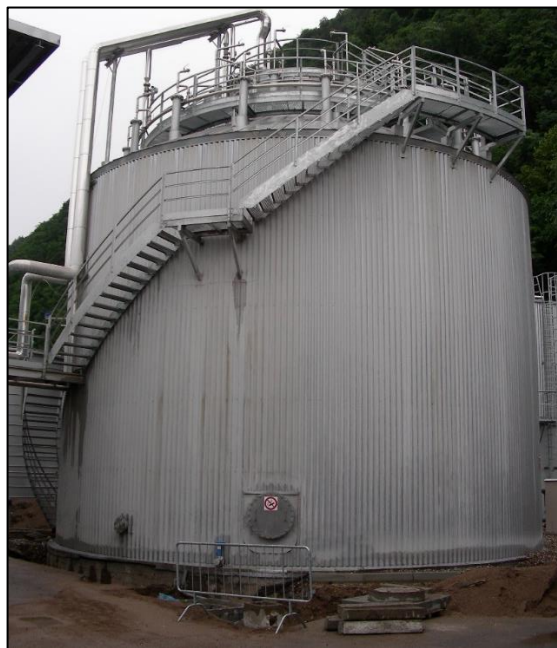
Picture 18: Upstream plug flow digester (UASB = up flow anaerobic sludge digester).
