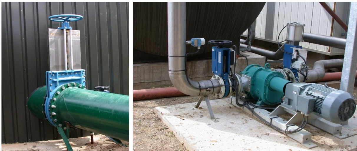
Picture 37: Rotary displacement pump with manually steered (left) and automatically steered (right) valve(s).
