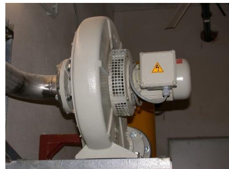
Picture 39: Radial fan.
