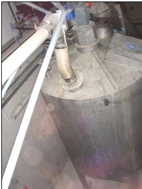
Picture 12: Substrate mixing tank followed by a feeding pump.
