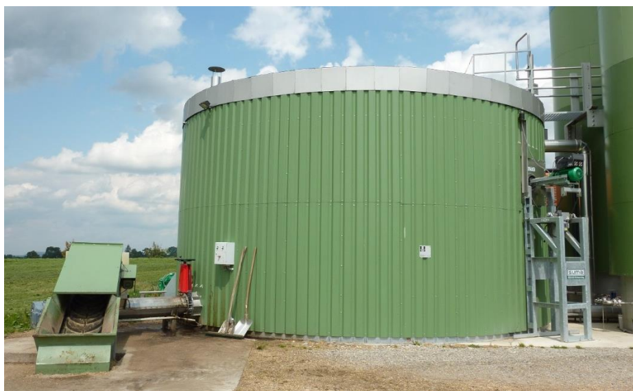
Picture 19: Hydrolysis tank upfront of the digester.
