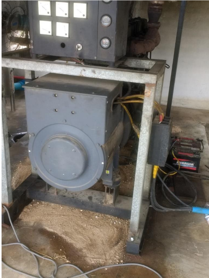
Unsafe Genset installation
