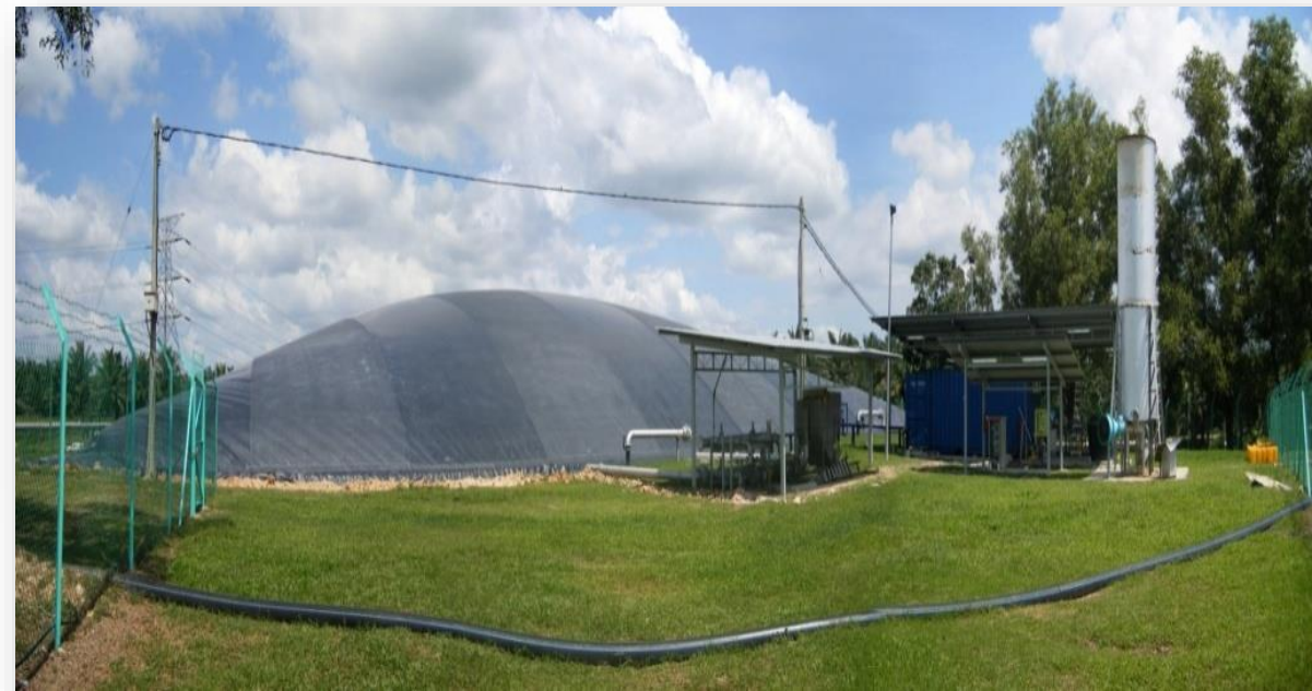
POME Biogas Power Plant, PTPN V, Kebun Tandun, Riau. Biogas: 850 m 3 /hour (60% CH 4 ). Capacity 1 MW
