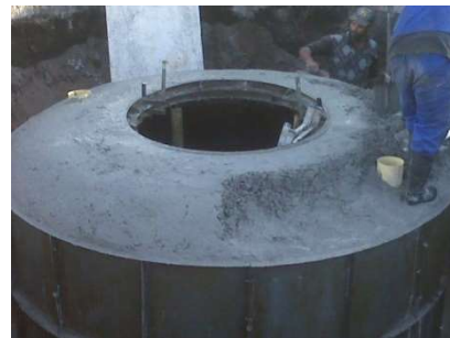
Brick & Mortar fixed dome digester
